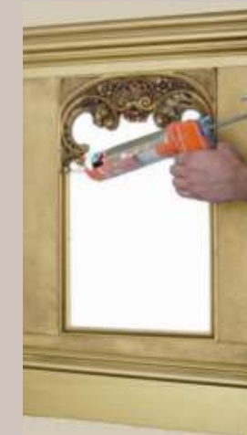
Caulk and fill all gaps, seams and joints. Spend time to do the job right. Caulk cleans up with a damp rag. Squeeze caulk through nozzle to fill gaps. Clean off excess with little finger and rag.
