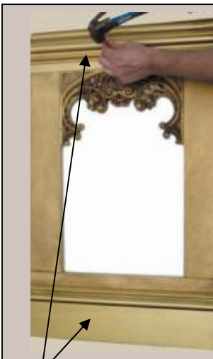
After panel tops & spacer boards are up, nail chair rail & base molding over MDF bases. Use adhesive caulk and a few finishing nails to attach each of the two moldings in place.
